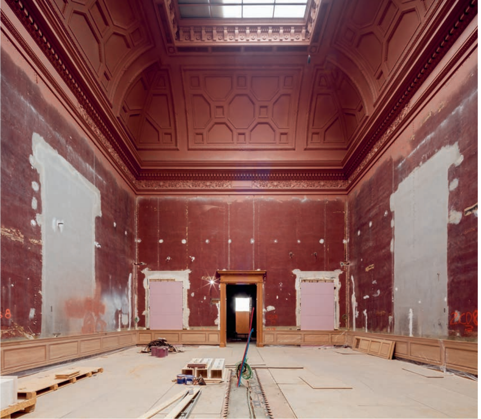
The two doorways to the Jordaens Gallery were replaced by one central doorway, returning it to its original state.
