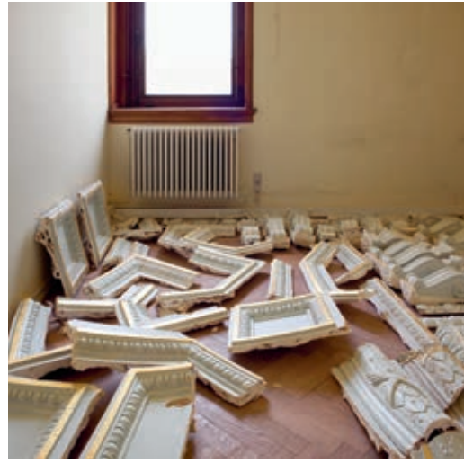
Ceiling mouldings were carefully stored and returned to their proper position later.
