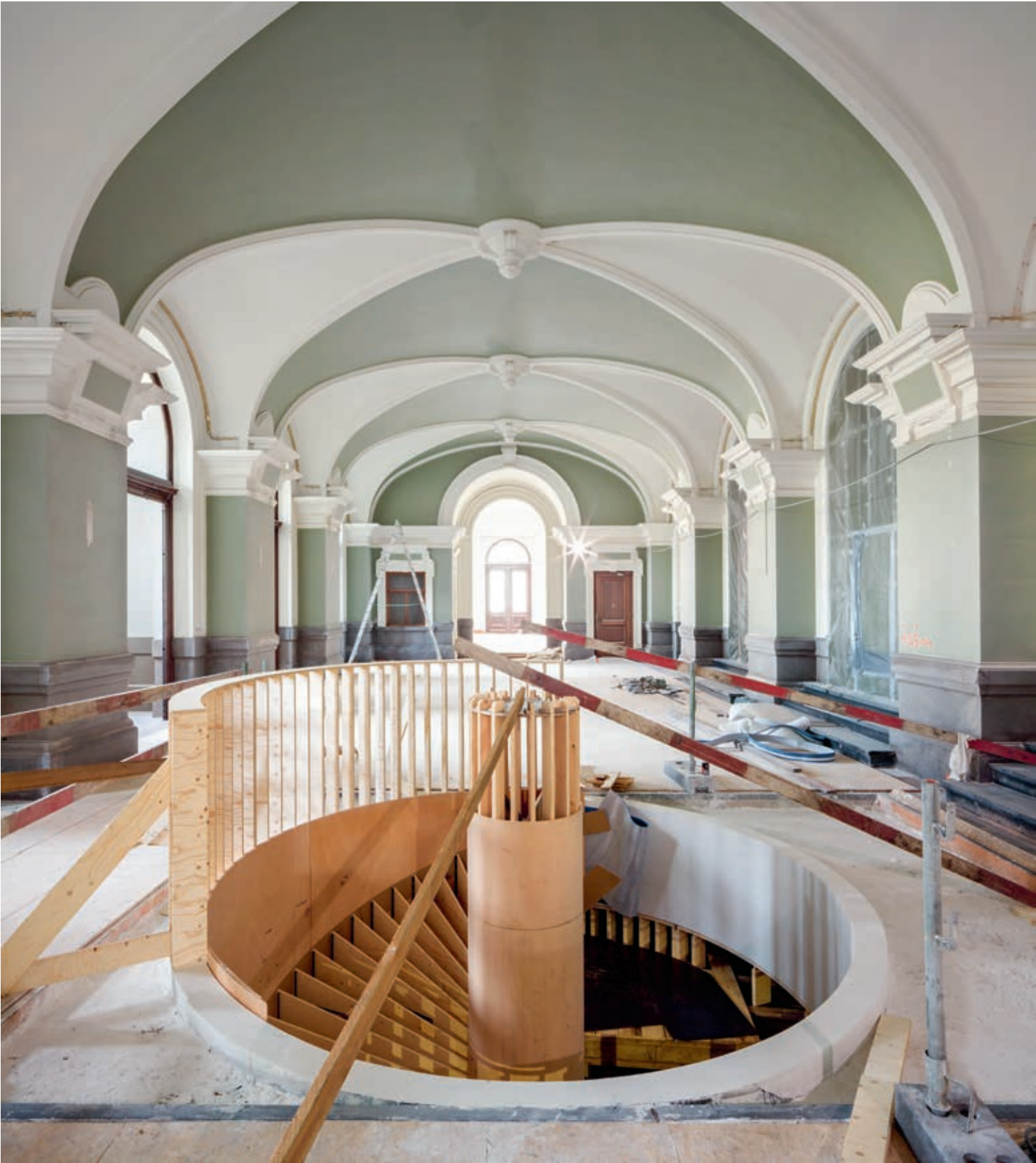
The concrete winding staircase in the entrance hall was cast in one piece.
