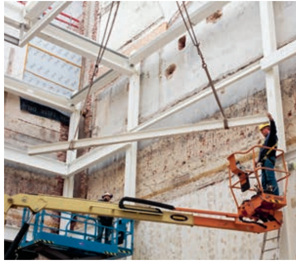
The patios are given a load-bearing steel structure weighing a million kilos.
