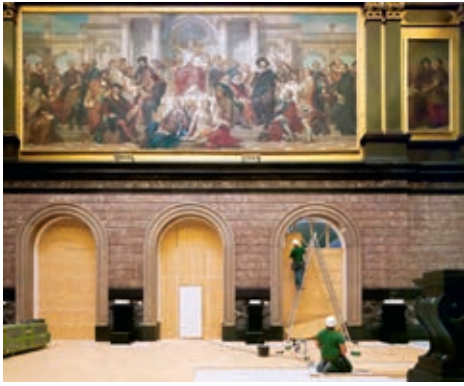
The De Keyserzaal was provided with a new gable roof but not renovated. The space was sealed and pressurised to keep it free of dust.
